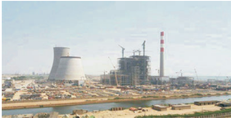
Sahiwal Coal fired power plant 9
