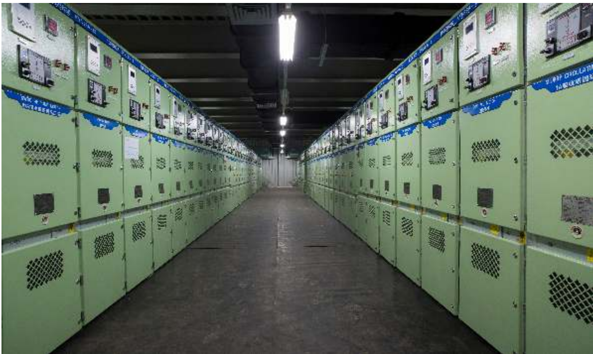
Installation of 11KV Distribution Cabinet
