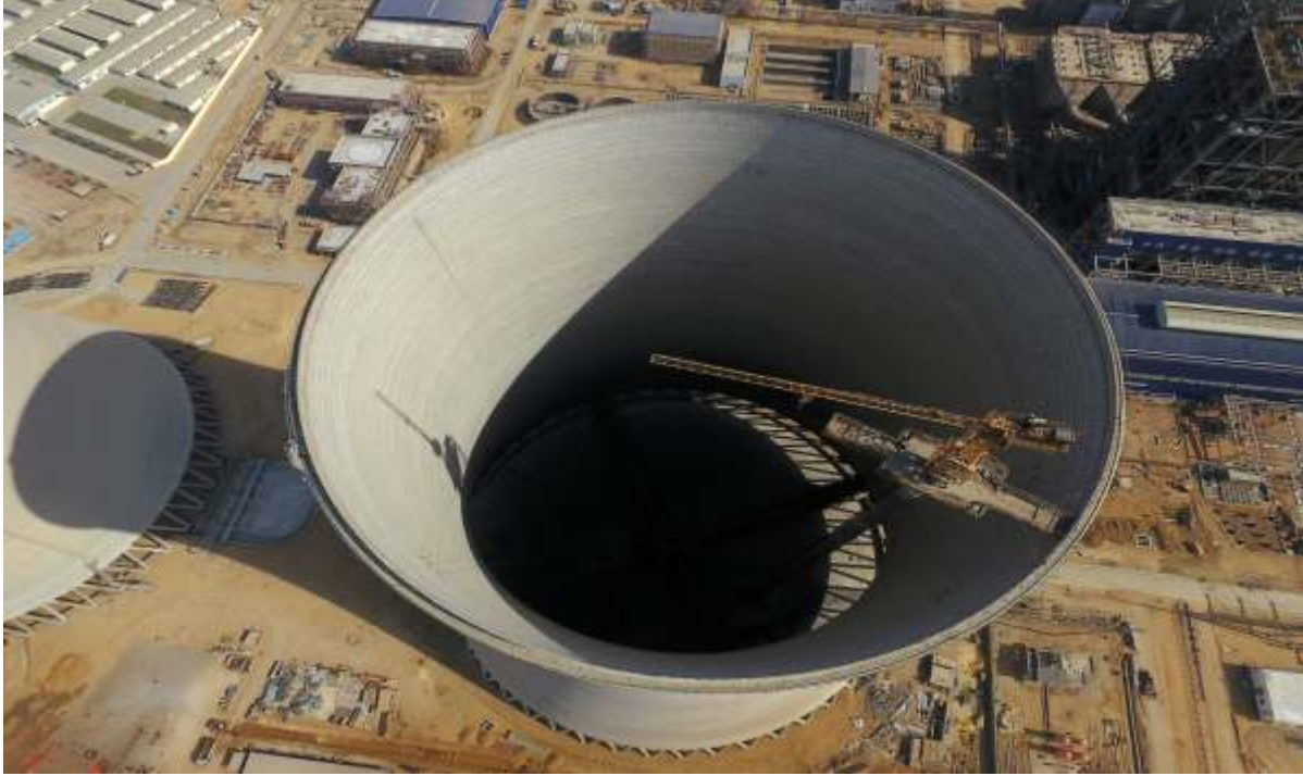
Cooling Tower Aerial View
